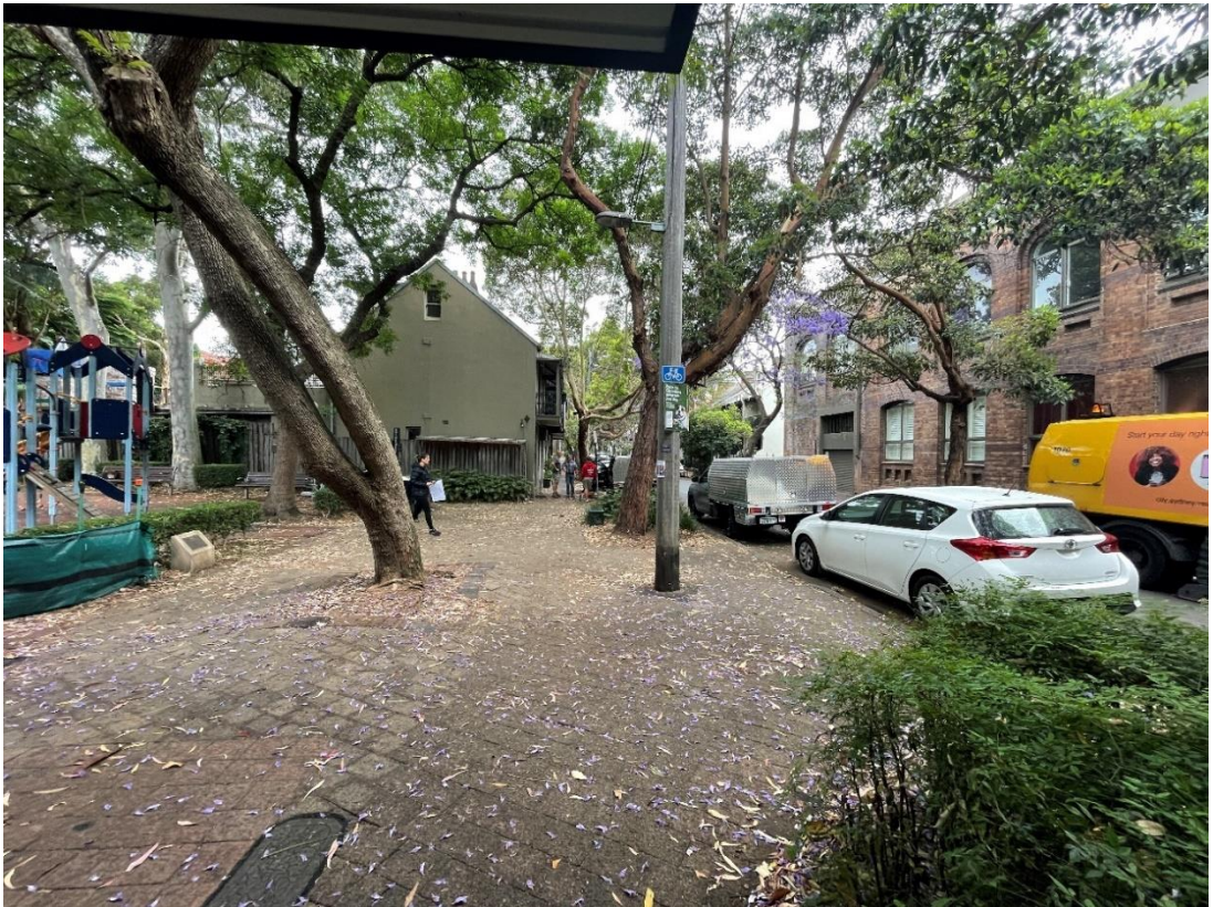
Looking south-east along Arthur Street – playground current location in the centre of the reserve. Uneven paving along the footpath.
